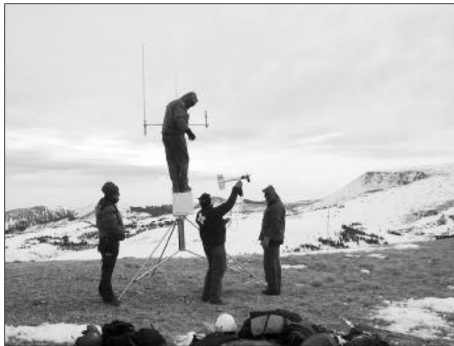
Chris McCollister, Dan Judd, Jim Farmer and Mike Rheam install the Mt. Coffin station, several miles north of Wyoming Peak in the Wyoming Range of the Bridger-Teton National Forest. At 10,800 feet this is the highest weather station in Wyoming. Photo by Bob Comey Bridger Teton National Forest Avalanche Center.
