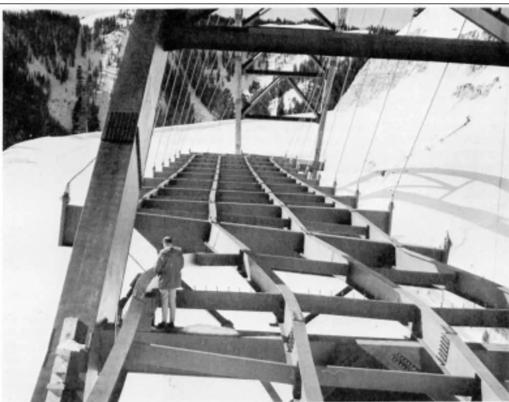
P-521811 On January 15, 1970, an avalanche twisted the steel girders of the unfinished bridge spanning over Glory Bowl's avalanche track. photo courtesy US Forest Service
