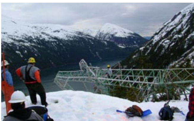
An avalanche April 16, 2008, on Crater Peak and Bride Peak near Juneau, Alaska, demolished Tower 3/5 and pulled over Tower 3/4. Cover photo by Mike Janes, inset photo by Eric Nielson
