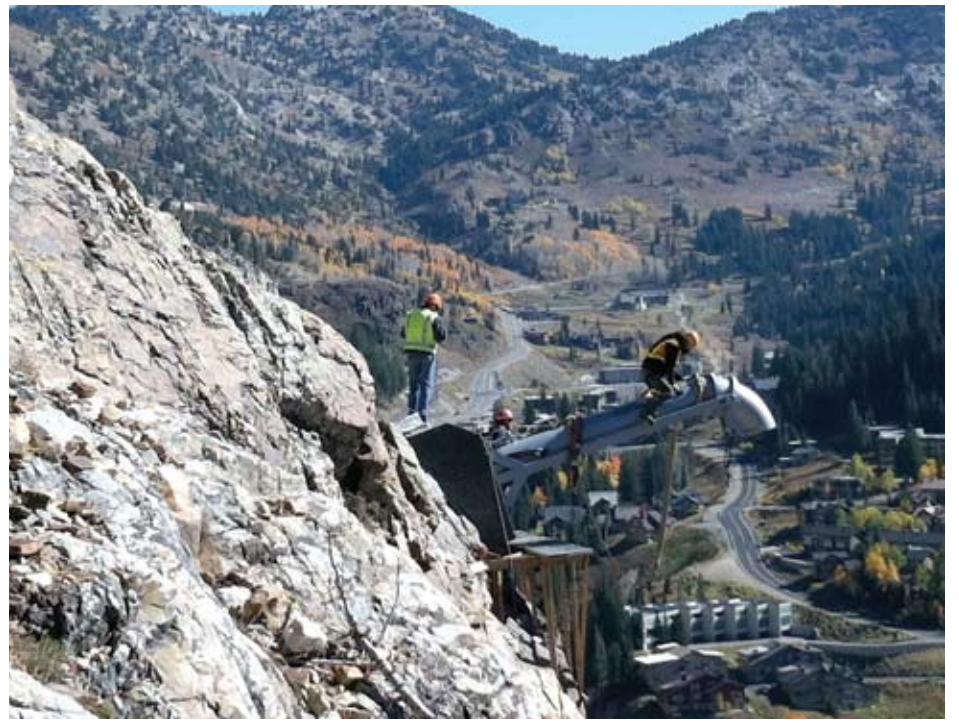
Doppelmayr USA, Inc., employees work on one of the two new Gazex installations.
