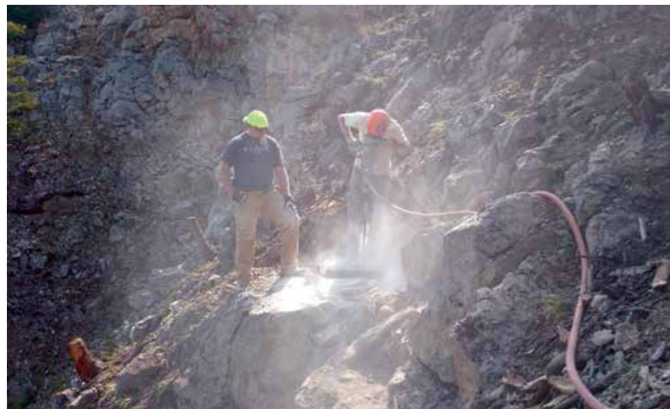
Drilling anchor bolts for O'bellx. (Surprisingly not the worst task we had.) Photo Brian Gorsage
