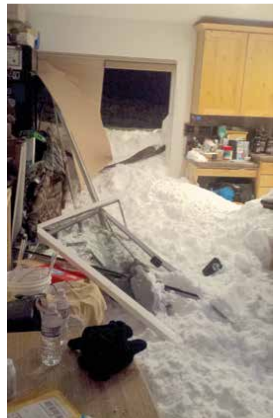
Eastern Sierra: McGee House in the McGee slide, side door to garage, door to kitchen. Photo Josh Feinberg
